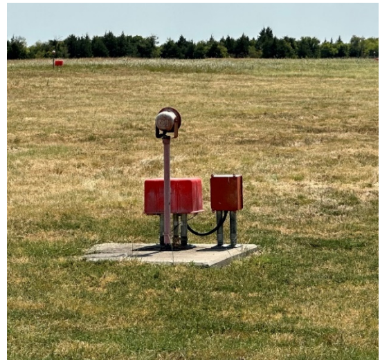
Runway End Identifier Light (REIL)
