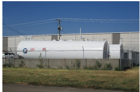
Jet A and 100LL Fuel Storage Tanks
