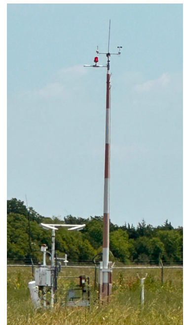
Automated Weather Observation System (AWOS)
