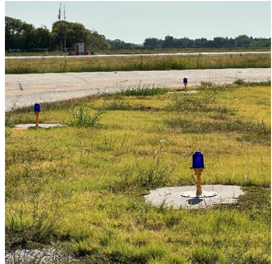
Medium Intensity Taxiway Lighting (MITL)
